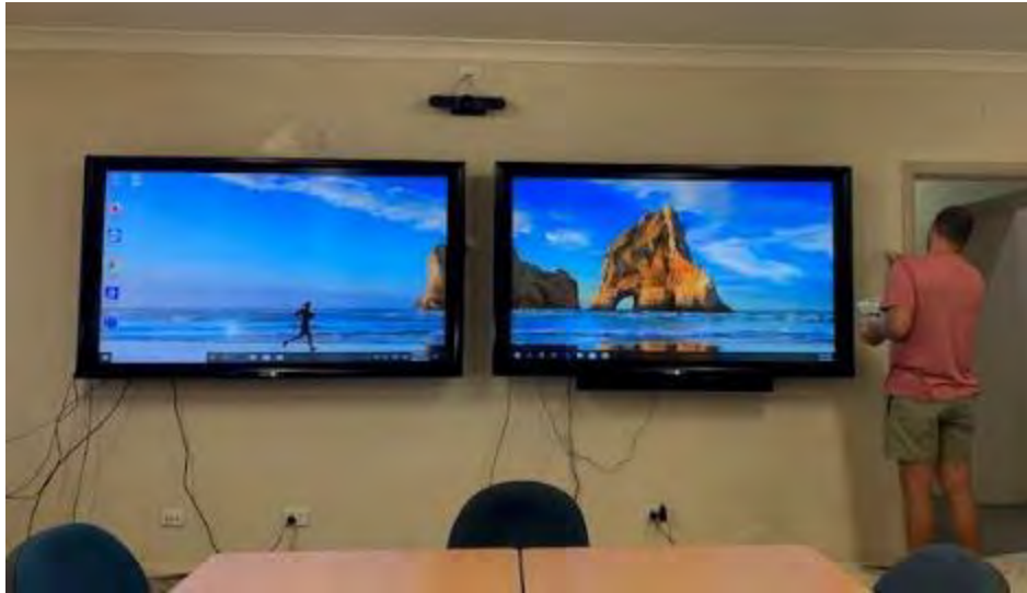
Tamworth Community College new IT infrastructure
